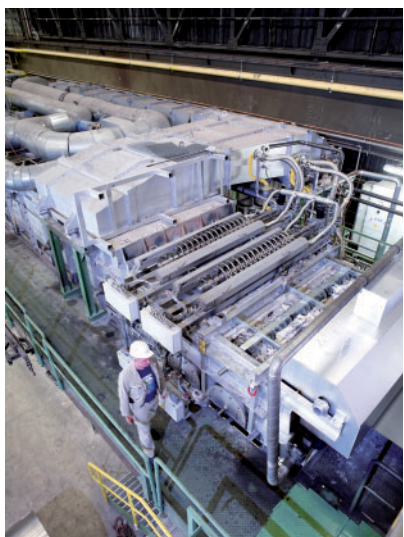
5 DFI Oxyfuel unit installed at Finntrop
