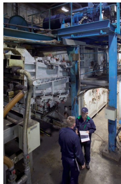
3 DFI Oxyfuel installation at entry side of stainless strip annealing line at Outokumpu, Nyby Works, Sweden
