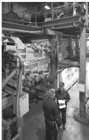
Figure 5: Compact DFI Unit at Outokumpu Nyby site
