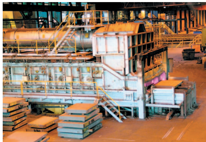
Walking beam furnace in Degerfors that has been converted to operation with REBOX-S flameless oxyfuel combustion technology.
