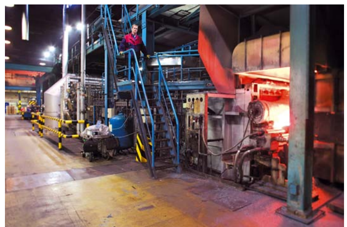
Catenary furnace in Nyby that has been converted to operation with REBOX-R flameless oxyfuel combustion technology. The furnace length remained unchanged, but production capacity was increased by 50 %.
