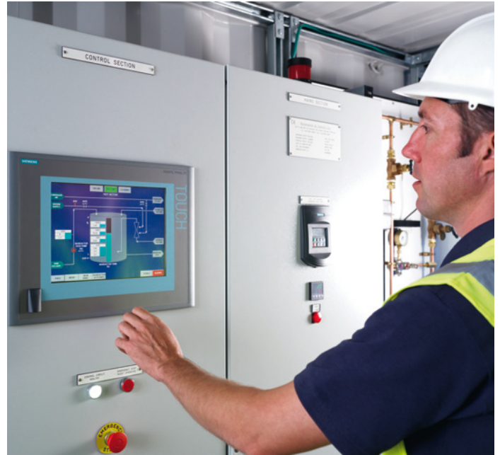
The AXENIS™ wastewater treatment system: easily monitored and controlled
