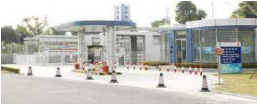
↑ Linde-designed first hydrogen refuelling station in Anting New Town Shanghai in 2009, with capacity to fuel three fuel-cell buses or 20 fuel-cell vehicles
